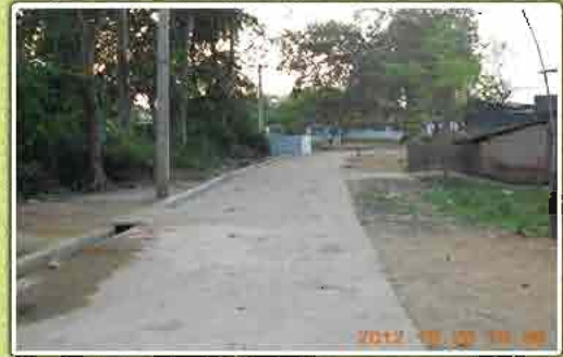
Construction of CC road with Drain & Garbage Bin at Ambapali Slum, ward No. 17.
